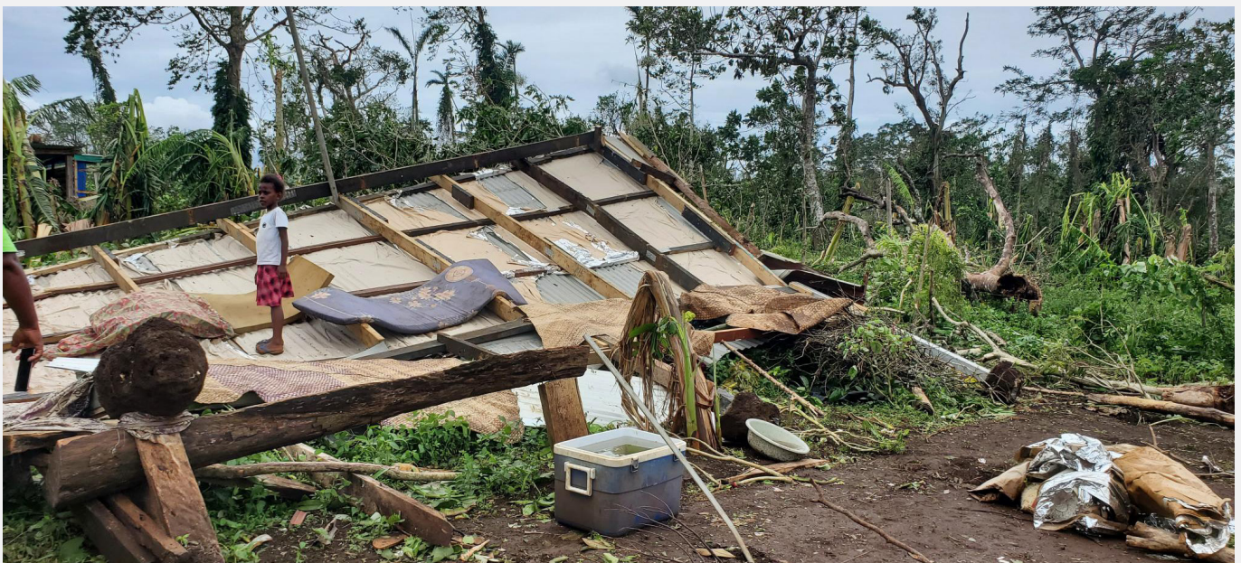
Tanna island was left with significant damage and limited communication after Tropical Cyclones Judy and Kevin made landfall within the same week in 2023.
